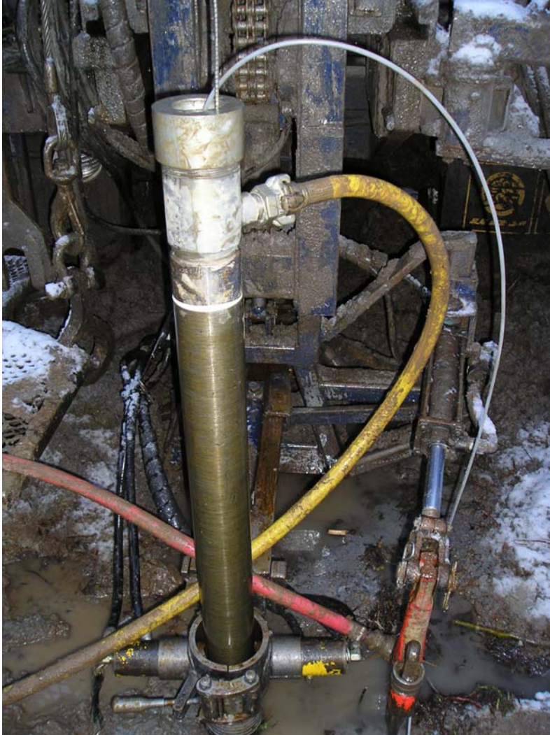
Photo I-19 Stuffing box used to seal the top of the drill pipes. The yellow hose pumps water into the interval being tested. The clear tube is the packer inflation hose.
